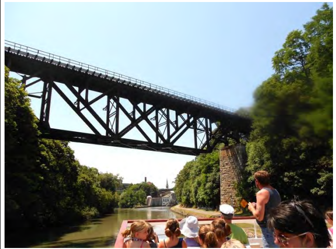
Upside-down RR Bridge
